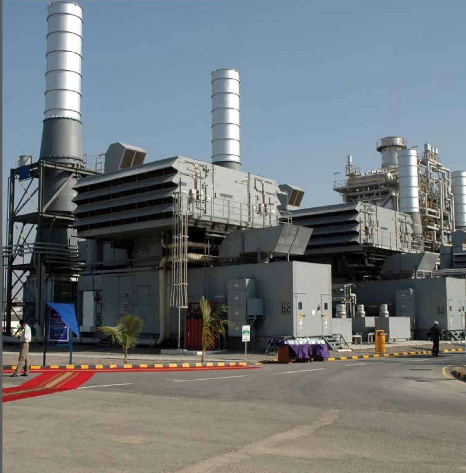
Korangi Combine Cycle Power Plant 220 MW
