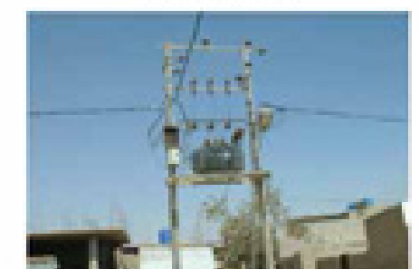
Post ABB Installation PWT
